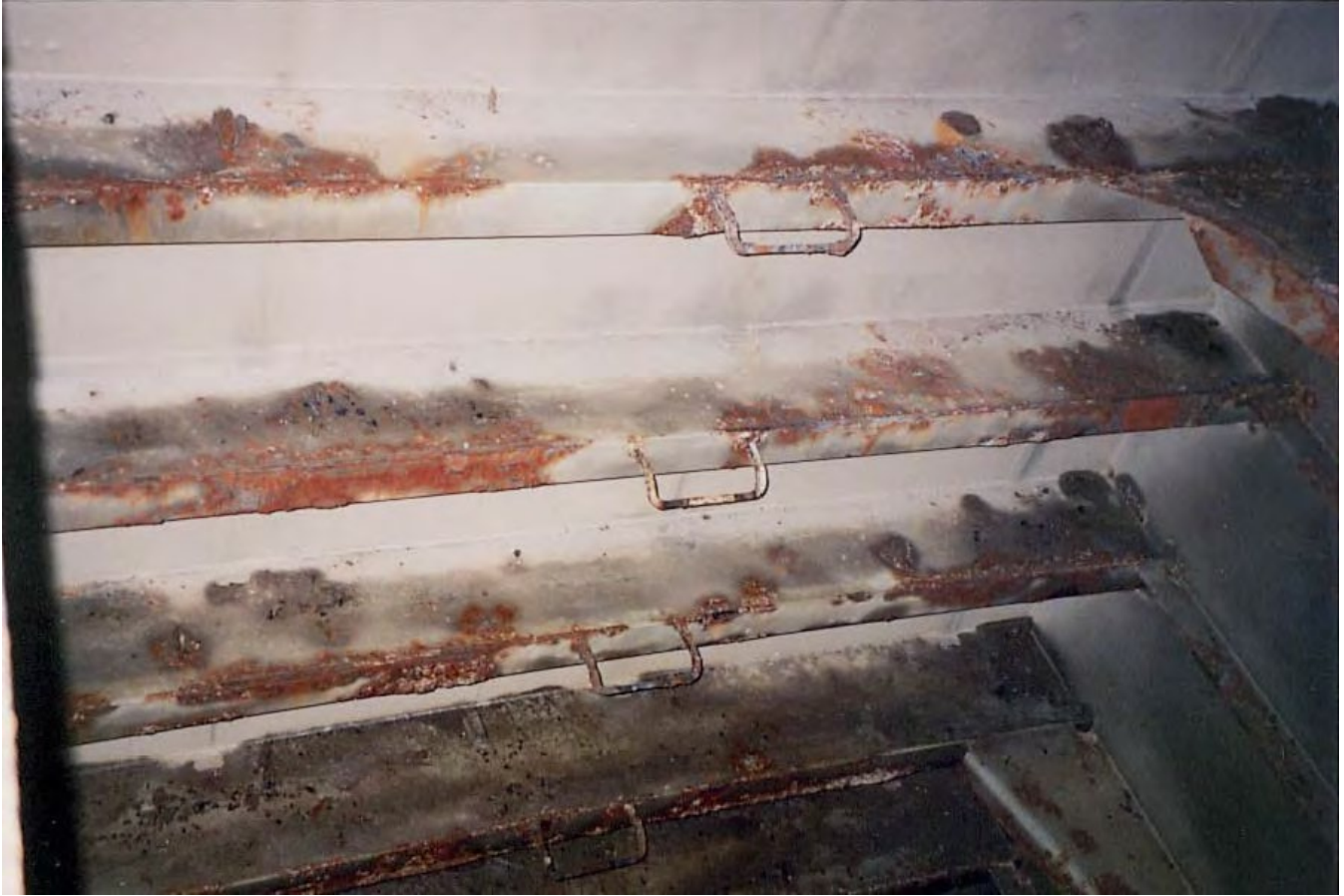
Fair Coating Condition
