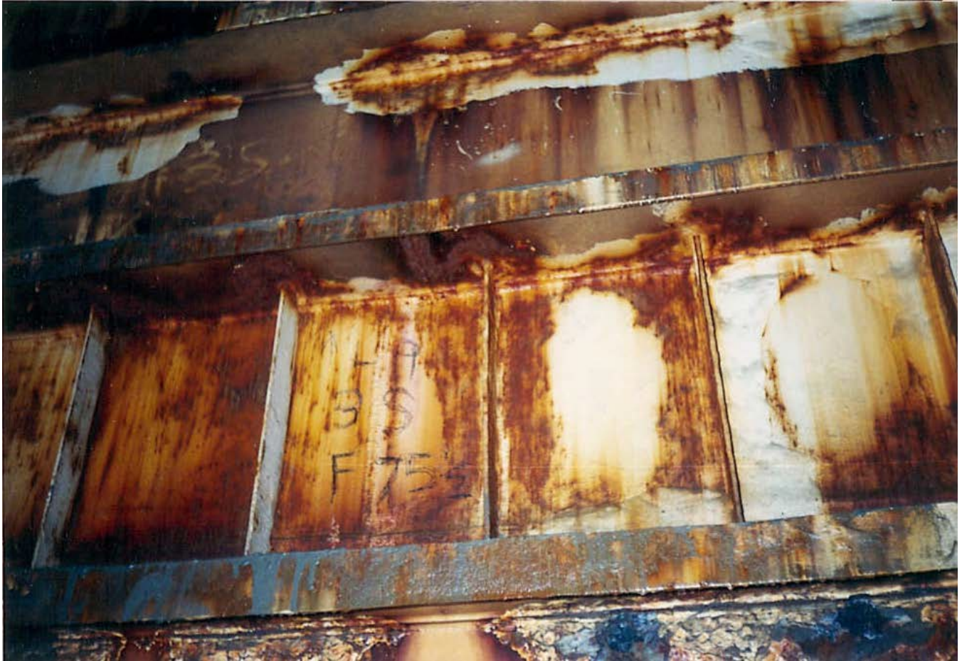
Poor Coating Condition
